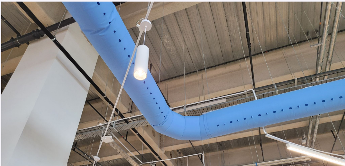
Figure 8. Textile air distribution ducts applied in a building.
